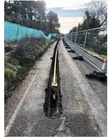
SGN Gas Works
